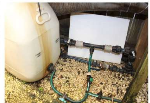
The 20 L supply tank and connections
